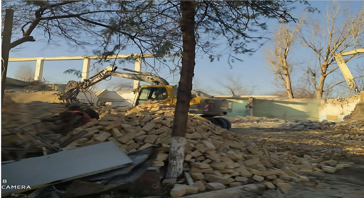
Fig.2. Not using enclosures in construction site
